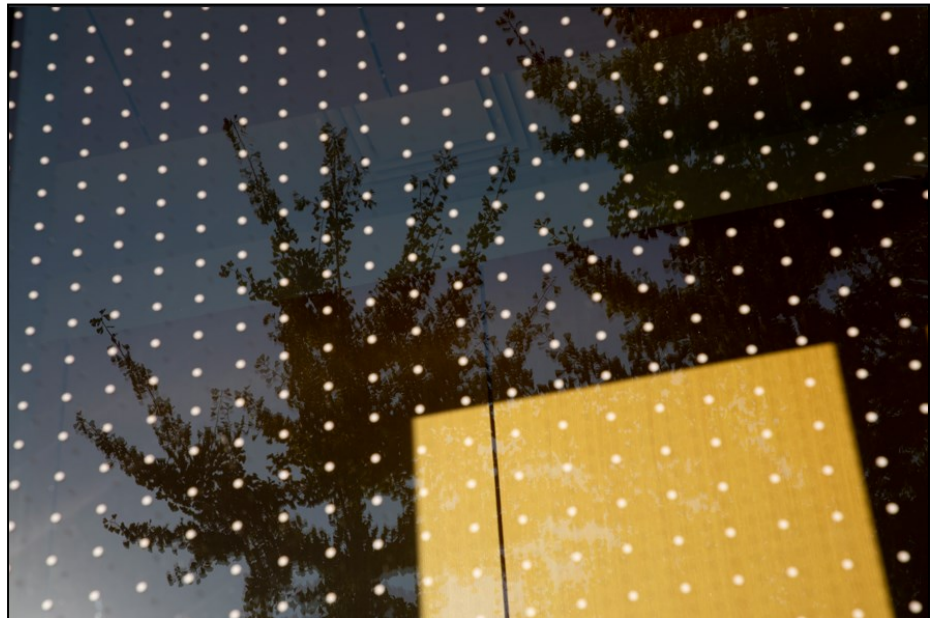
Bird-friendly glass along an inner courtyard of Lauder College House at the University of Pennsylvania in Philadelphia, Pennsylvania, October 21, 2021. The window decals are used to break up the reflections birds see to prevent window collisions. Photo: Luke Franke, Audubon.
